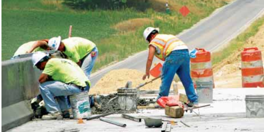
Southwest Indiana stands to benefit from improved access to jobs, education and health care with I-69. Pictured, crews pour sidewall on S.R. 61 interchange bridge in Pike County.
