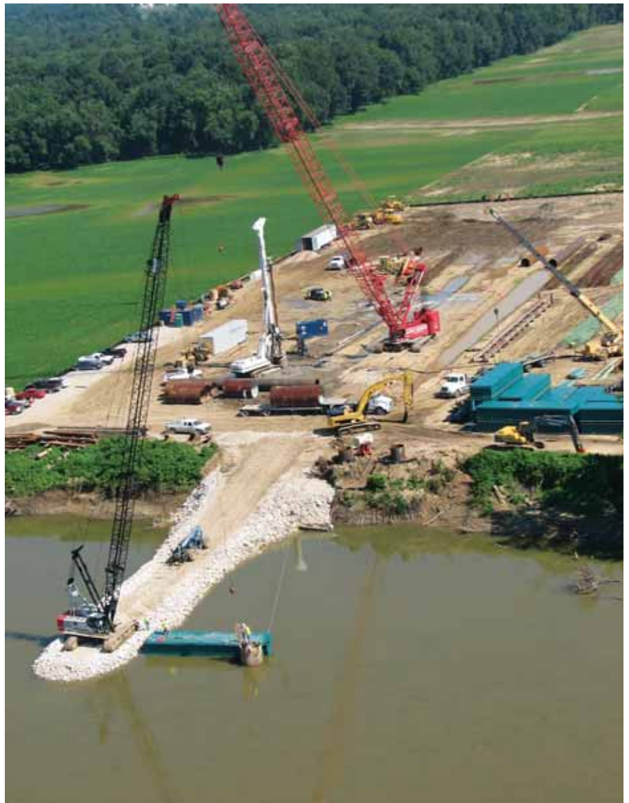
Top left: Paving asphalt ramps at S.R. 64 interchange in Gibson County. Top: I-69 bridges over the White River on the Pike-Daviess county line. Above: Aerial photo of White River bridge construction on the Pike-Daviess county line.
